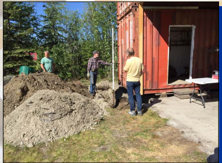
Checking the depth of the holes. The backhoe could only get part way. Lots of hand digging was provided by the volunteers.
