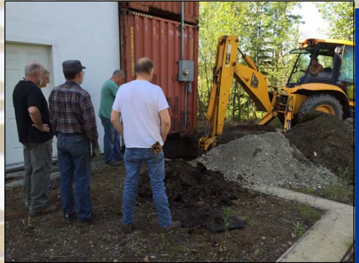
Some of the volunteers for Saturday's workday watch the backhoe at work on the northwest corner.
