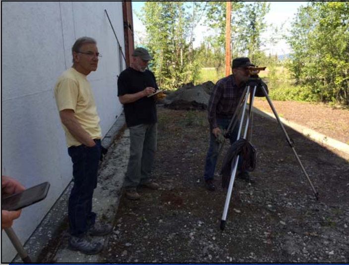
Matt, Michael and Bill check the survey stake behind the hangar to verify the depth of the foundation holes.
