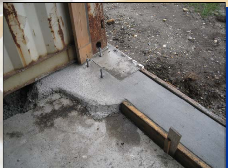
At the end of the new sill we've put in anchor bolts to hold the door vertical side rails.
