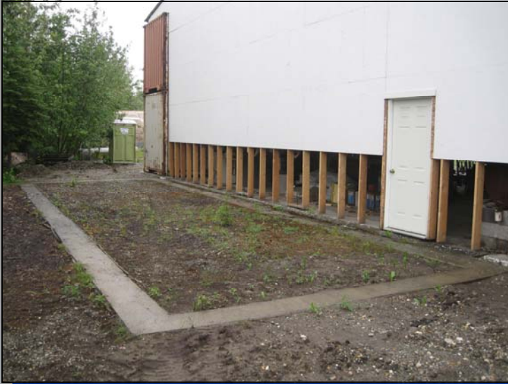
Footing on the back of the hangar - might be a great place to build a heated meeting area?
