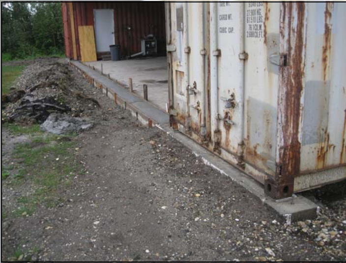
Conexs sitting on the new concrete foundations. Also the new concrete sill for the door is in place.
