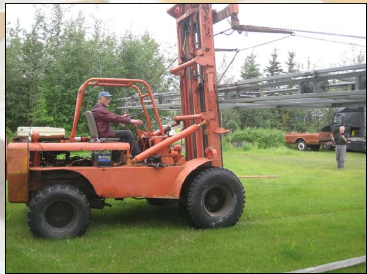
Syd at the controls with Terry guiding as the door is lowered onto some wood blocking
