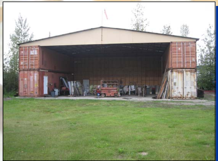
Front wall has been removed so that the door header can be installed.
